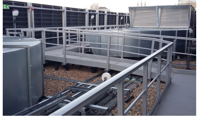
Emergency Disabled Roof Access Ramp
